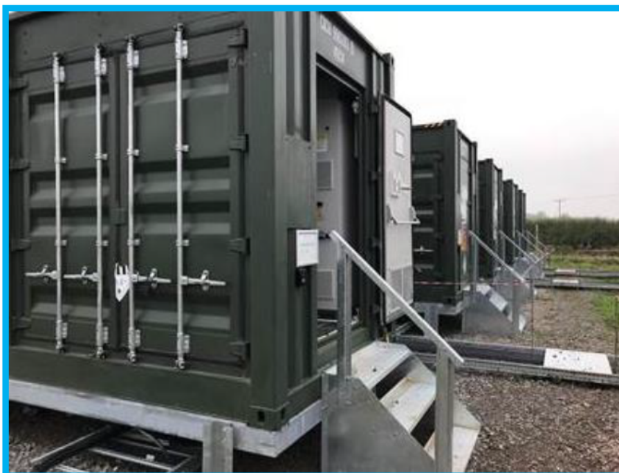
Fig 22 Typical containerised batteries on legs with permeable gravel base below.
