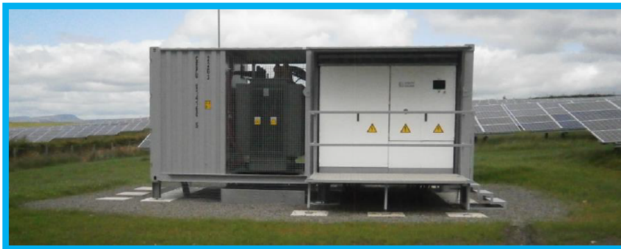
Fig 21 Typical transformer unit on legs over permeable gravel bed.
